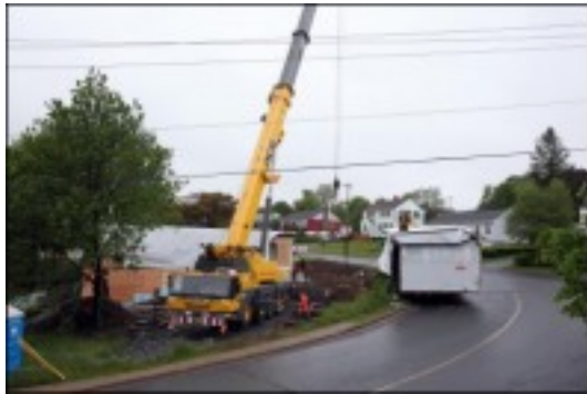
Photo: Workers prepare to lift a second section of a modular home on to its foundation at Lakecrest Drive in Dartmouth. (Eric Wynne / Staff)
